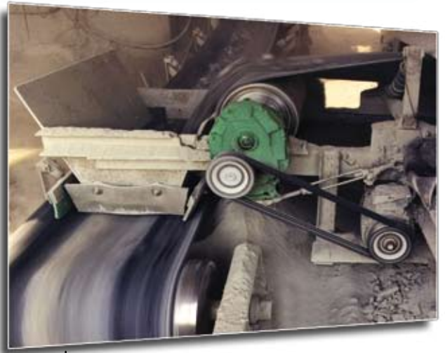
► Belt conveyor drive
